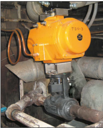
A Velan Power Ball valve in service.
