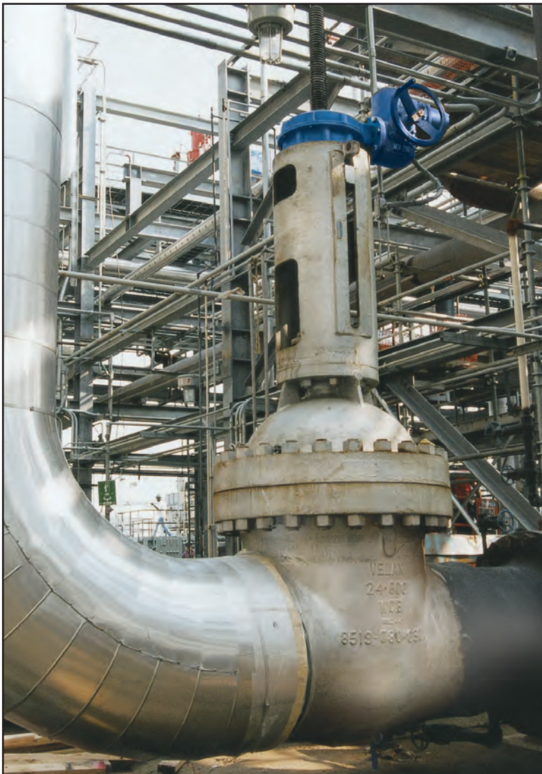
Carbon steel gate valve, ASME Class 600 used for boiler feed water installation at a hydrogen plant in Texas.
